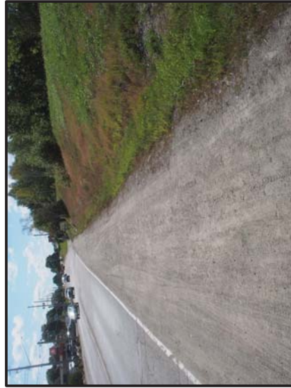
Image 6. Photograph 487 showing the gravel shoulder and a disturbed drainage feature.
