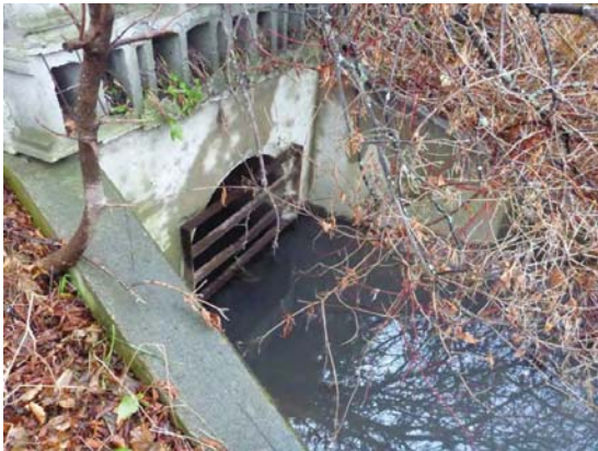
Plate 3: Storm sewer outlet at unnamed watercourse. Headwall and culvert to be replaced (November 26, 2015).
