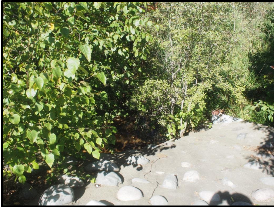
Image 23. Photograph 629 showing boulder-embedded concrete in the disturbed creek bed.
