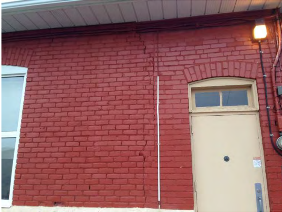
Figure 5: Vertical crack at south elevation. Original brick on left side of crack; infill brick to the right.
