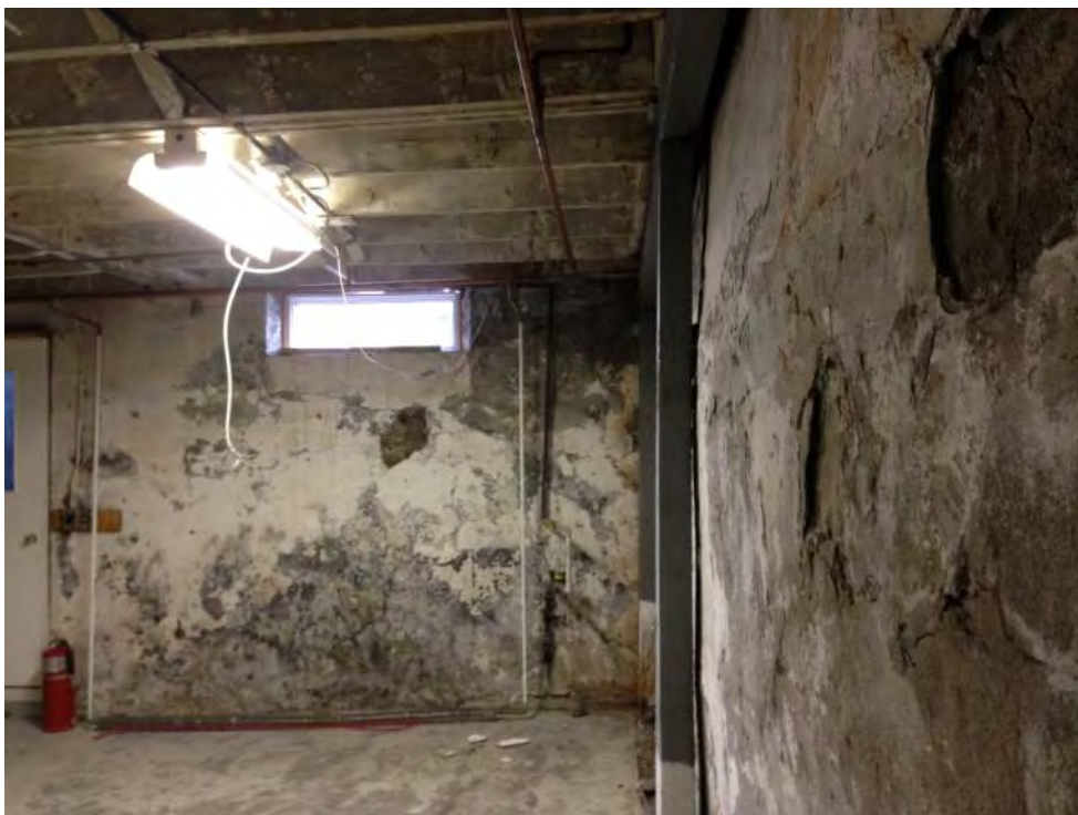
Figure 12: Concrete foundation walls are bowing inward.
