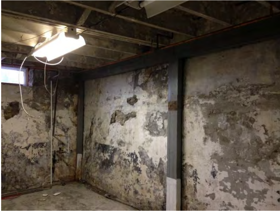
Figure 11: Concrete foundation walls cracking and spalling below grade.
