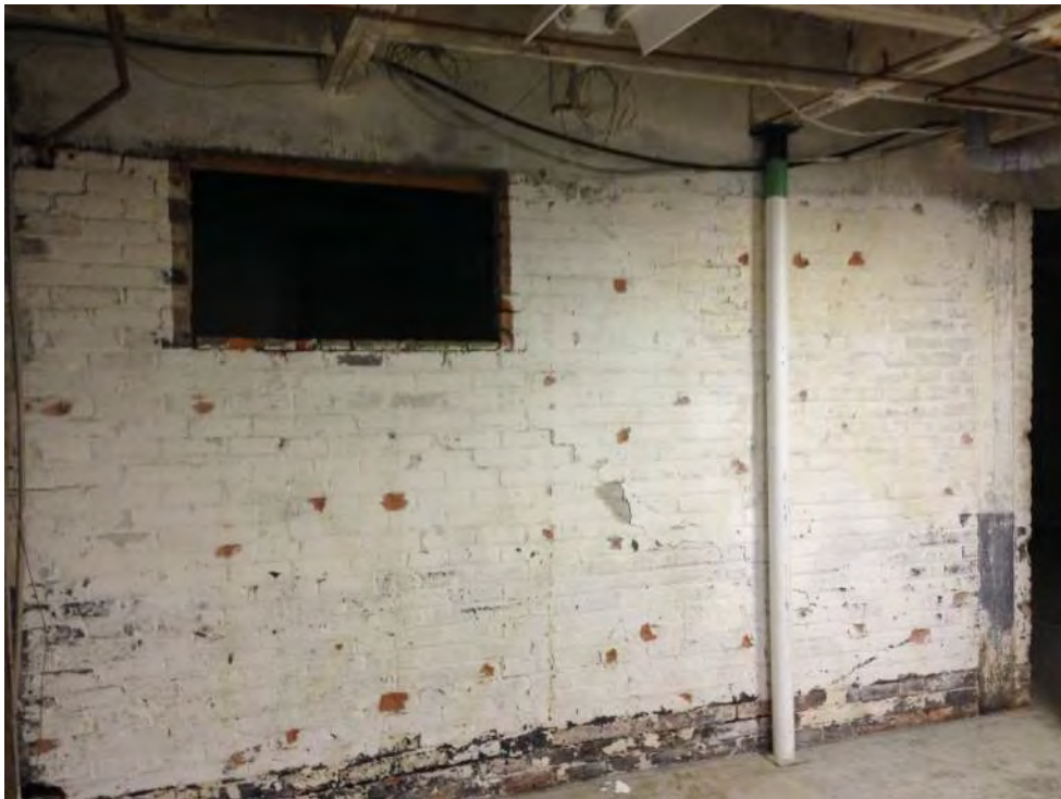
Figure 14: Typical deteriorated condition of load-bearing brick walls in basement.
