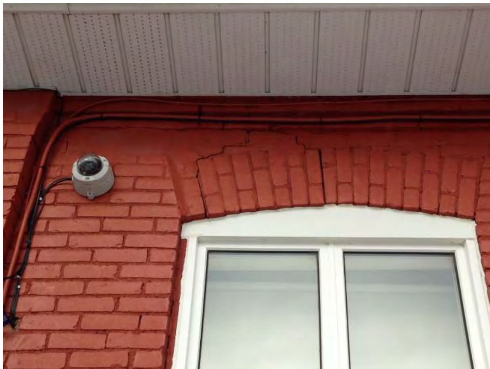
Figure 4: Typical brick masonry cracking at original arched window lintels.
