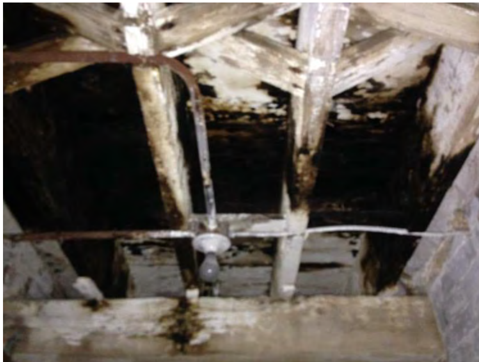
Figure 10: Fire damage to wood joists in basement corridor.
