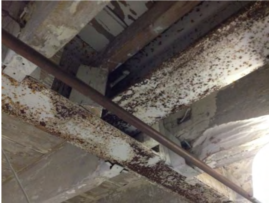
Figure 9: Typical steel beam surface corrosion.
