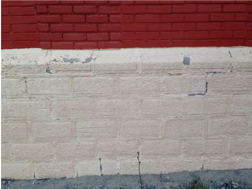
Figure 13: Typical concrete block foundation wall cracking above grade.
